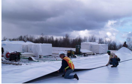
The new roof will be fully completed once the front façade of the building is done.
